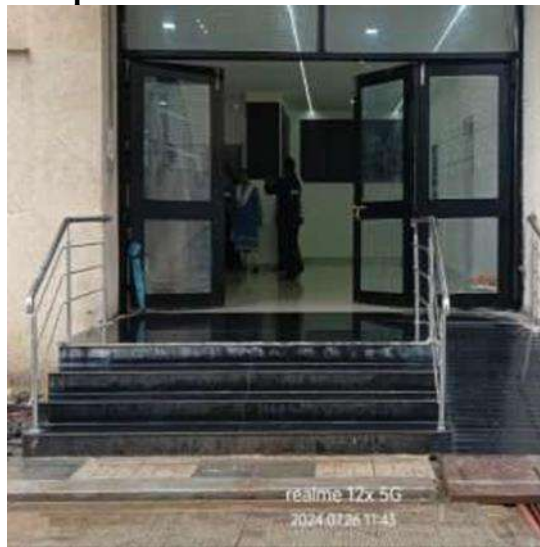
Ramp – Barrier free environment
