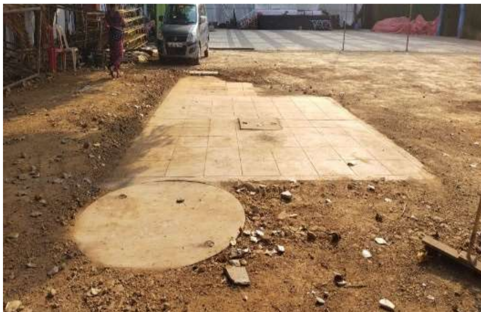
Rain Water Harvesting Units
