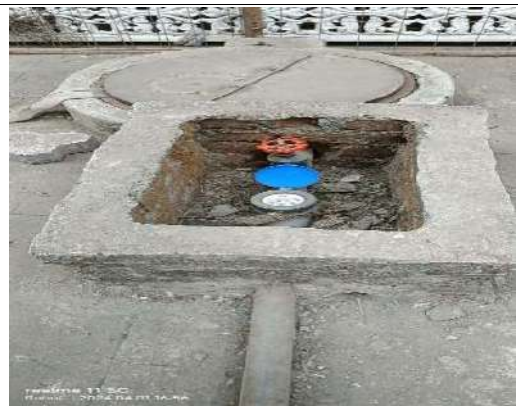
Water Management System on campus
