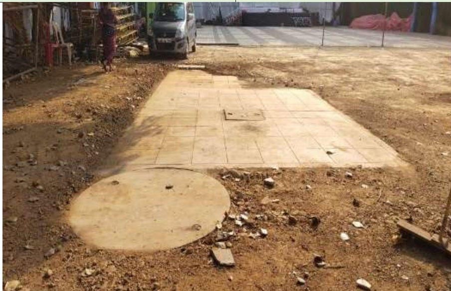
Rain Water Harvesting Units
