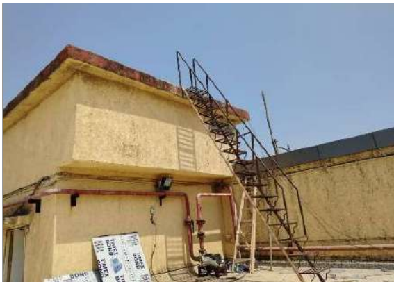
Water Management System on campus
