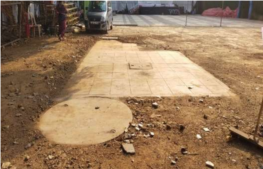
Rain Water Harvesting Units
