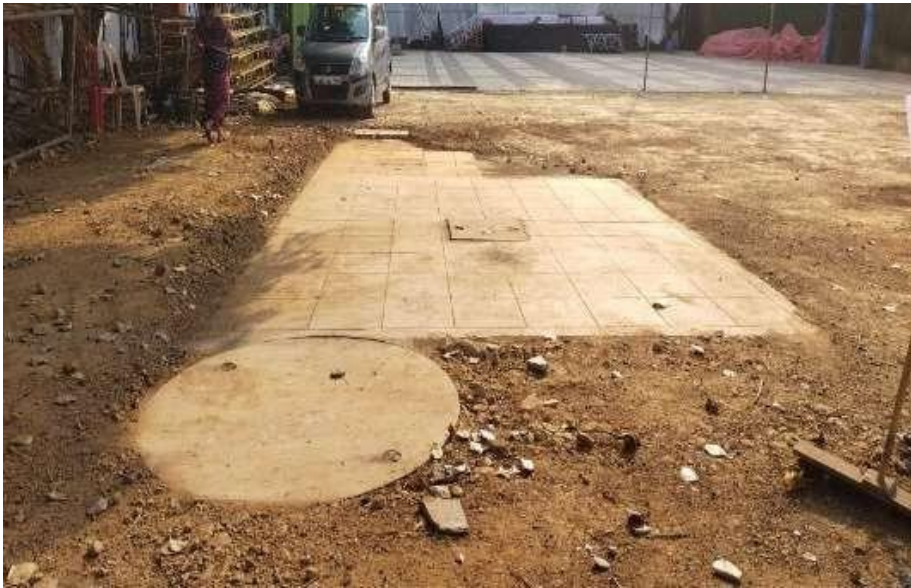
Rain Water Harvesting Units
